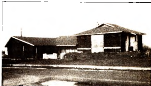
The Nazarene church parsonage, adjacent to the historical marker, under construction, March 1983.
